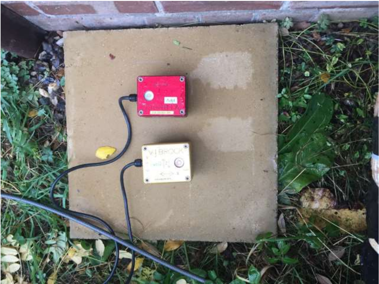
Figure 4.2: Vibration monitoring equipment installed at The Old Railway Gatehouse on the closest façade to The Street
